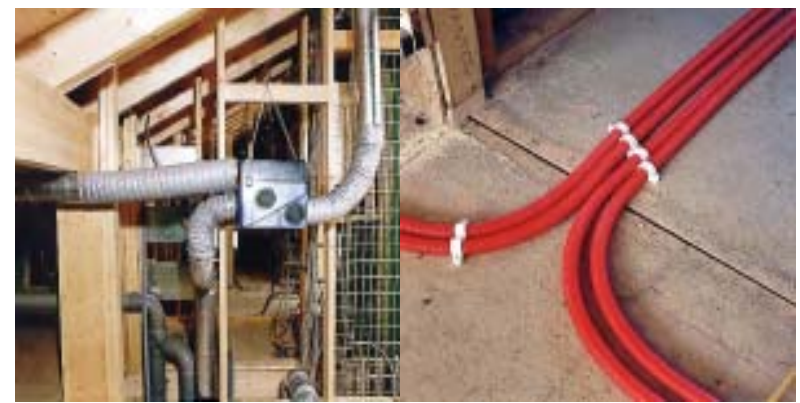
INTEGER Millennium House - Building services
